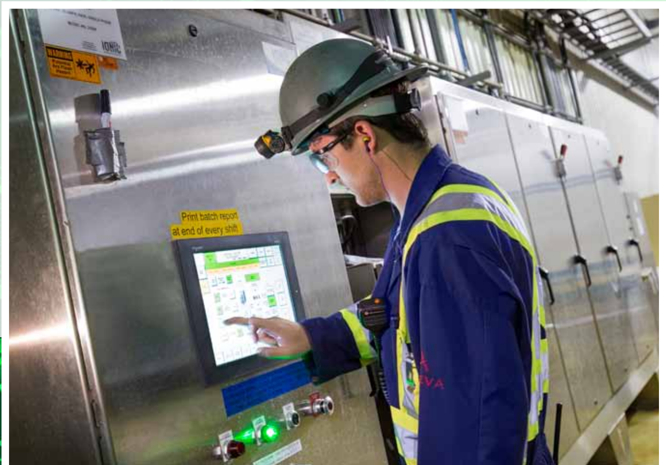
An Orano employee uses a control panel in the yellowcake packaging area.
