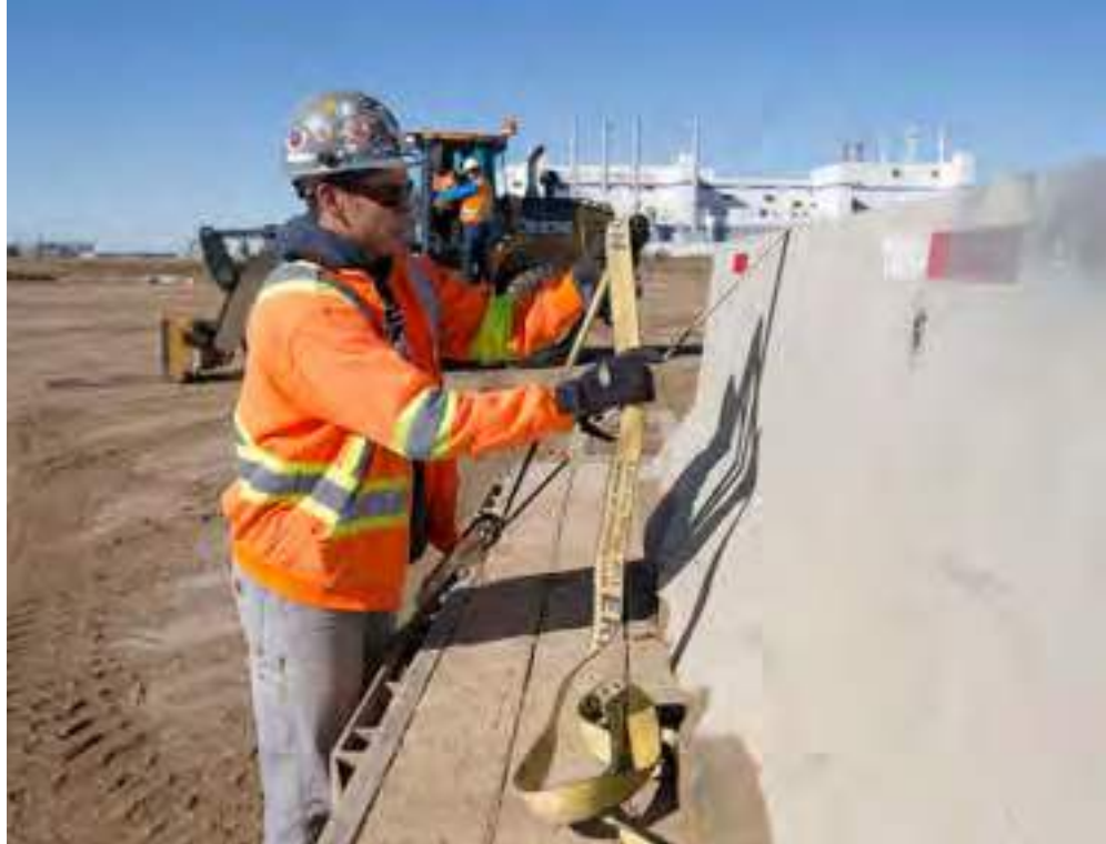
An employee from the Walters Alberici Joint Venture works on a construction project at K+S’s Bethune Mine. Photo Courtesy of K+S Potash Canada.
